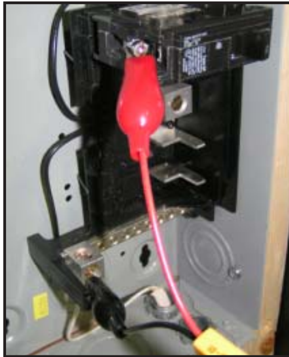
Test Lamp on Circuit Breaker
