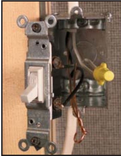
Copper Wires Ready for Connection
