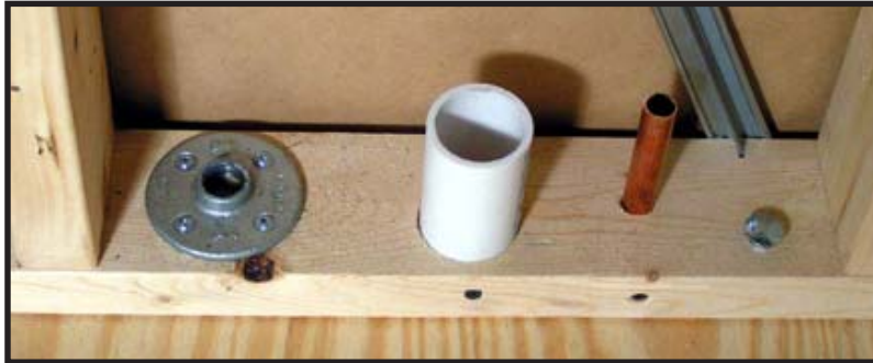
Three Pipe Connections in Sole Plate
